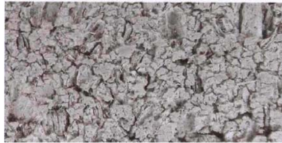
Figure 3. Surface cracking and micro-cracking due to exposure to ultraviolet radiation
